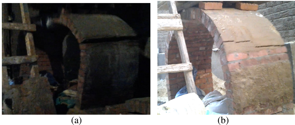
Figure 14 Mode of failure for vaults strengthened by (a) ferro-cement wire mesh, b) Polyester mortar
